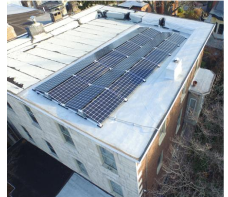
Solar on a row home (Solar States)
